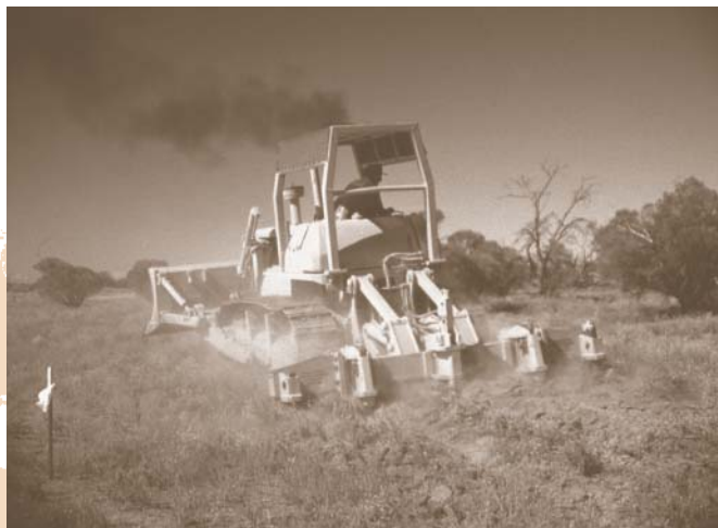
THE USE OF HEAVY MACHINERY WITH MULTIPLE TINES AND WINGED BOOTS GENERALLY INCREASES THE EFFICIENCY OF RIPPING OPERATIONS
